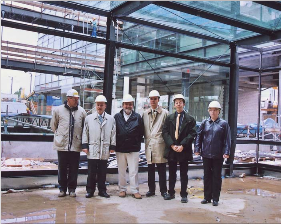
V isit to the building site of the new training centre of the “Chambre de Commerce” (FORMCHCO II project)
